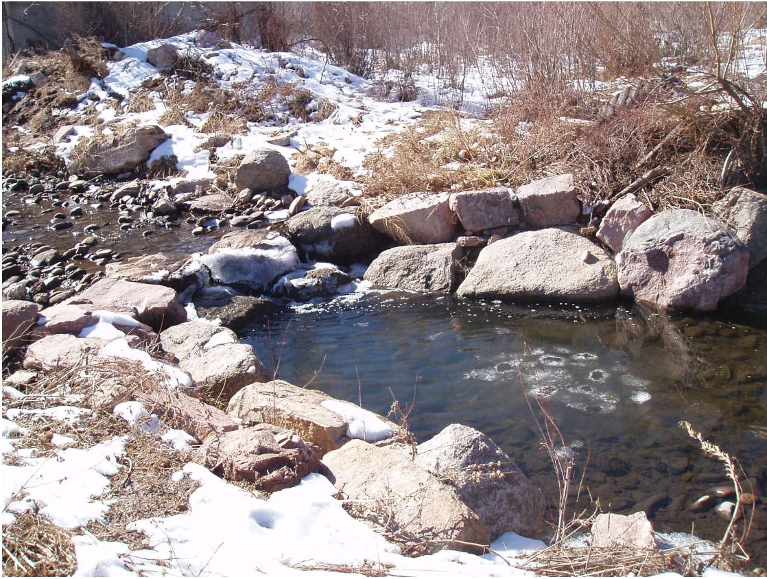
Cross Vane Structure on Cheyenne Creek below I-25 Overpass. Colorado Springs, El Paso County, Colorado
