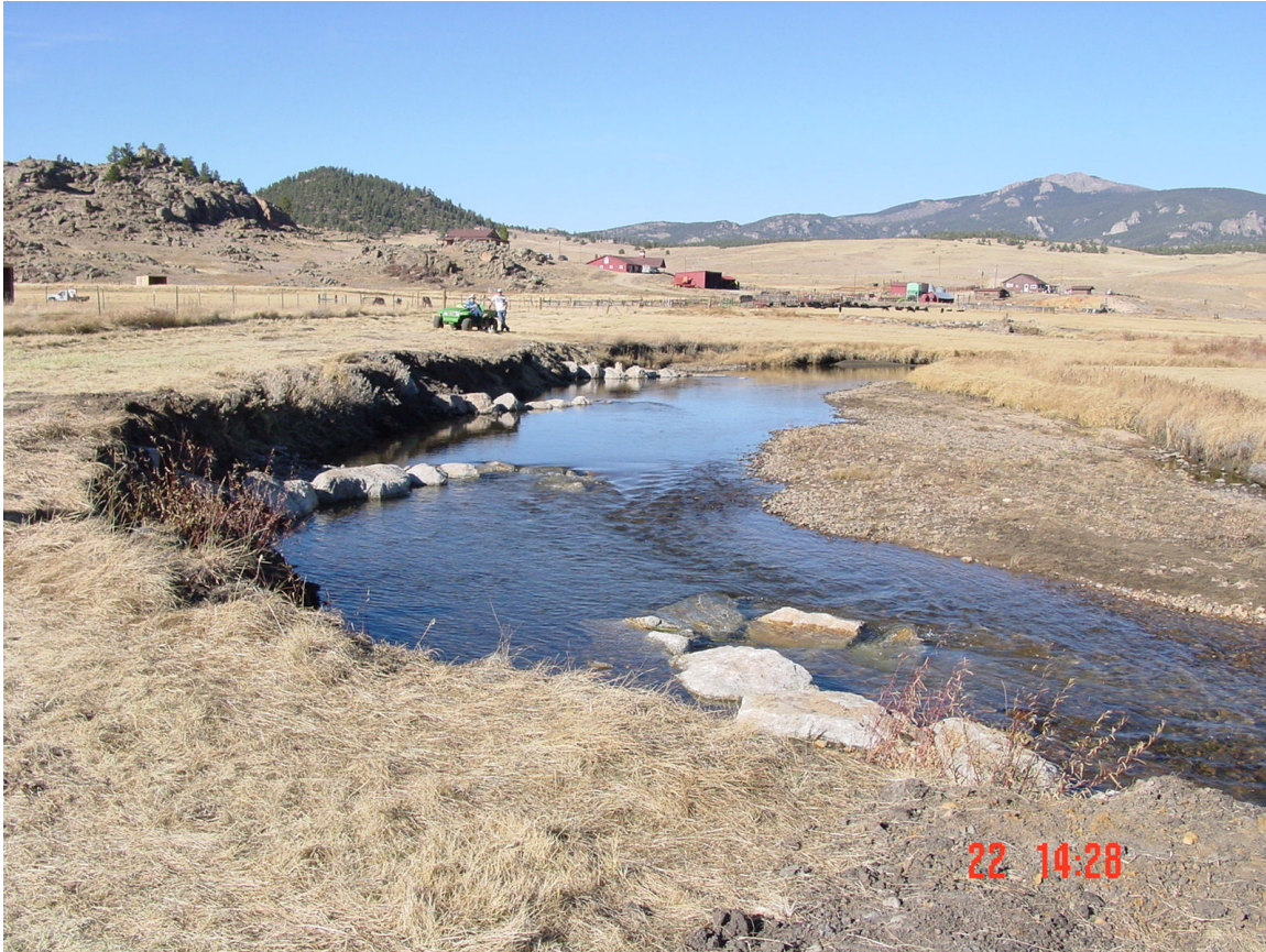
Eagle Rock Ranch - Rock J-Hook Vanes installed to protect stream banks and adjacent road,, 2003.
