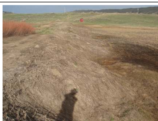
Photo 12: Eroding Downstream side of Dam.
