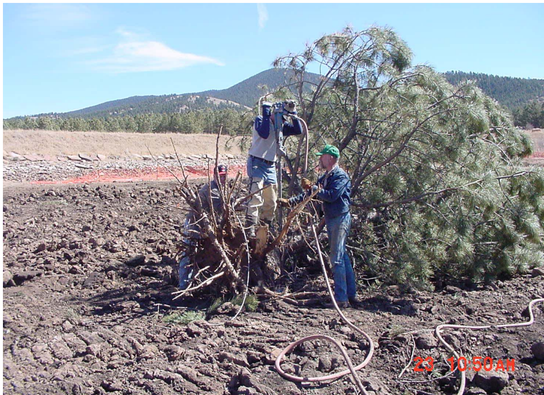
Photo 7: Trout Unlimited volunteers anchor a large pine in the lake bottom using a 90lb pneumatic drill and stainless steel Manta-Ray MR-1 anchors. Manitou Lake, Teller County, CO.
