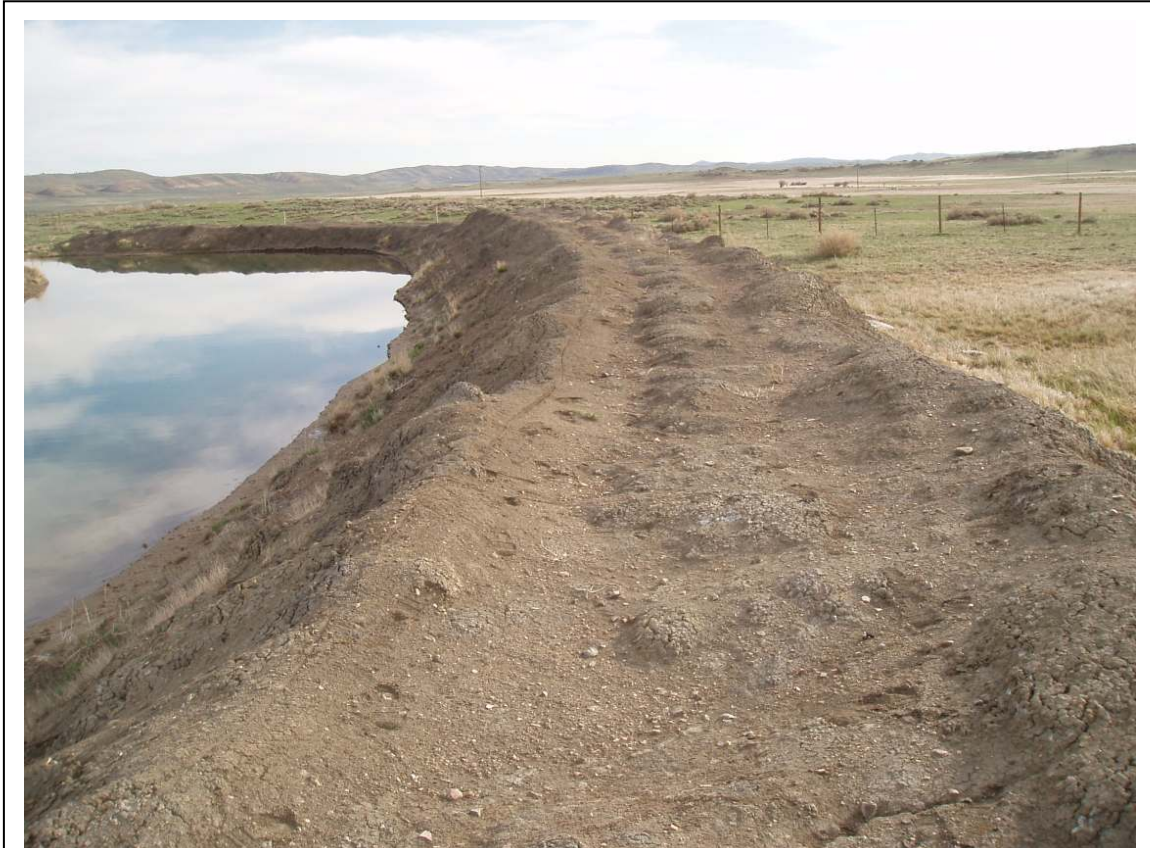
Photo 2: Spoils Pile and Eroding Bank at Eagle Lake.
